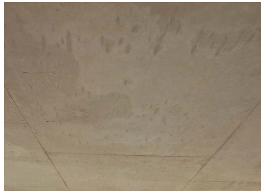
Rippling effect on concrete.
