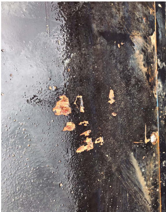
Mark left on the face of the panel by the vibrator.
