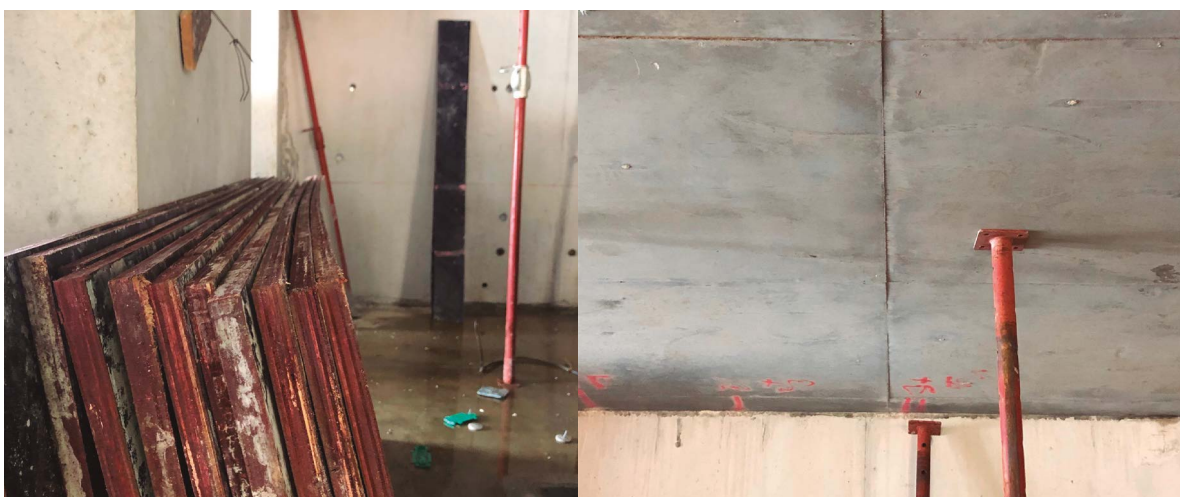
Incorrect shoring between panels.
