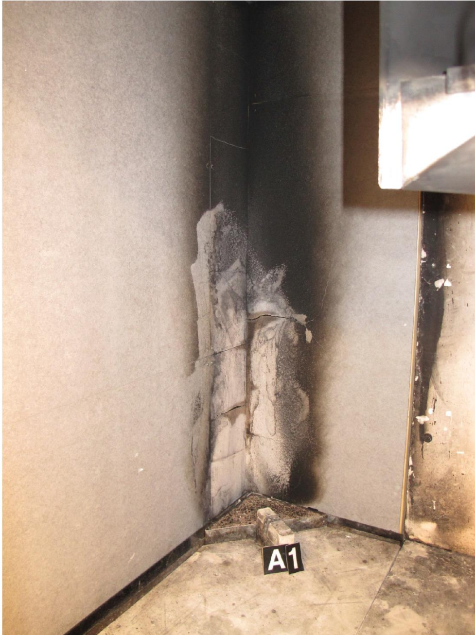
Photo no 3 After test “Fibersementplate BF”
