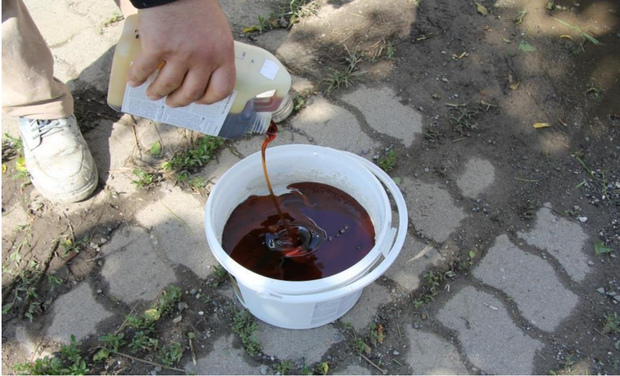
4. Prepare polyurethane adhesive, pour it onto the substrate, and apply with fine serrated float (jag 2 mm).
