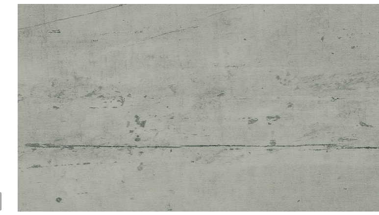
2585 Cold Cracked Concrete 177.8 x 1219.2mm
