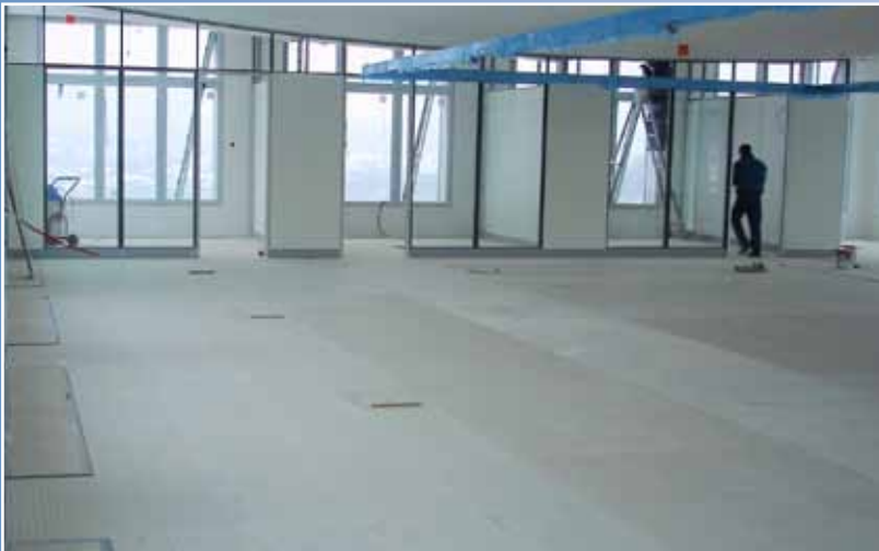
Barmenia Office Building - MERO hollow floor Combi T
