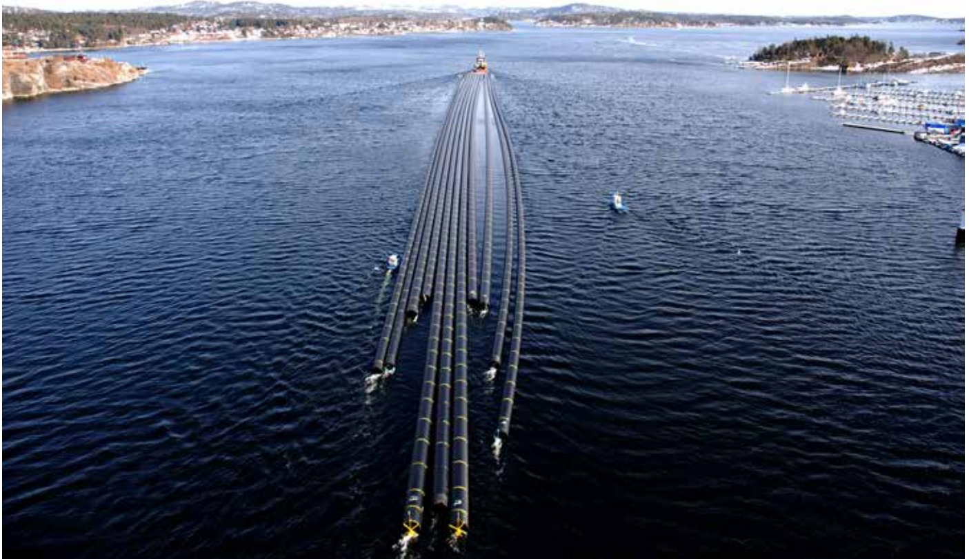
Picture 2 - Departure of eleven OD1600 and OD2100 mm pipes, lengths between 500-600m.
