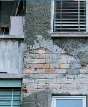
Degraded building facade in need of repair
